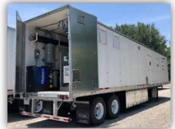
2400 High Vacuum Purifier with 300KW Sound Attenuated Generator and Dry Air System
